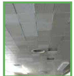
Deteriorating fencing and leaky roofs need repair or replacement
